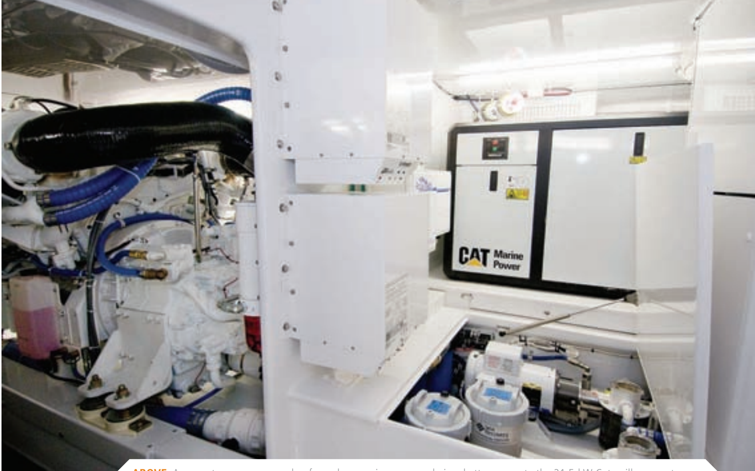
ABOVE: A separate pump room makes for a clean engine room and gives better access to the 21.5-kW Caterpillar gensets.
